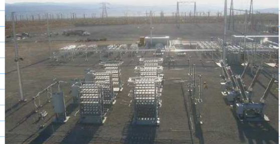
500 kV shunt Capacitor Banks
